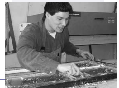
New 89 Lexington Ave. tenant Chris Eastman works on restoring a wood window
